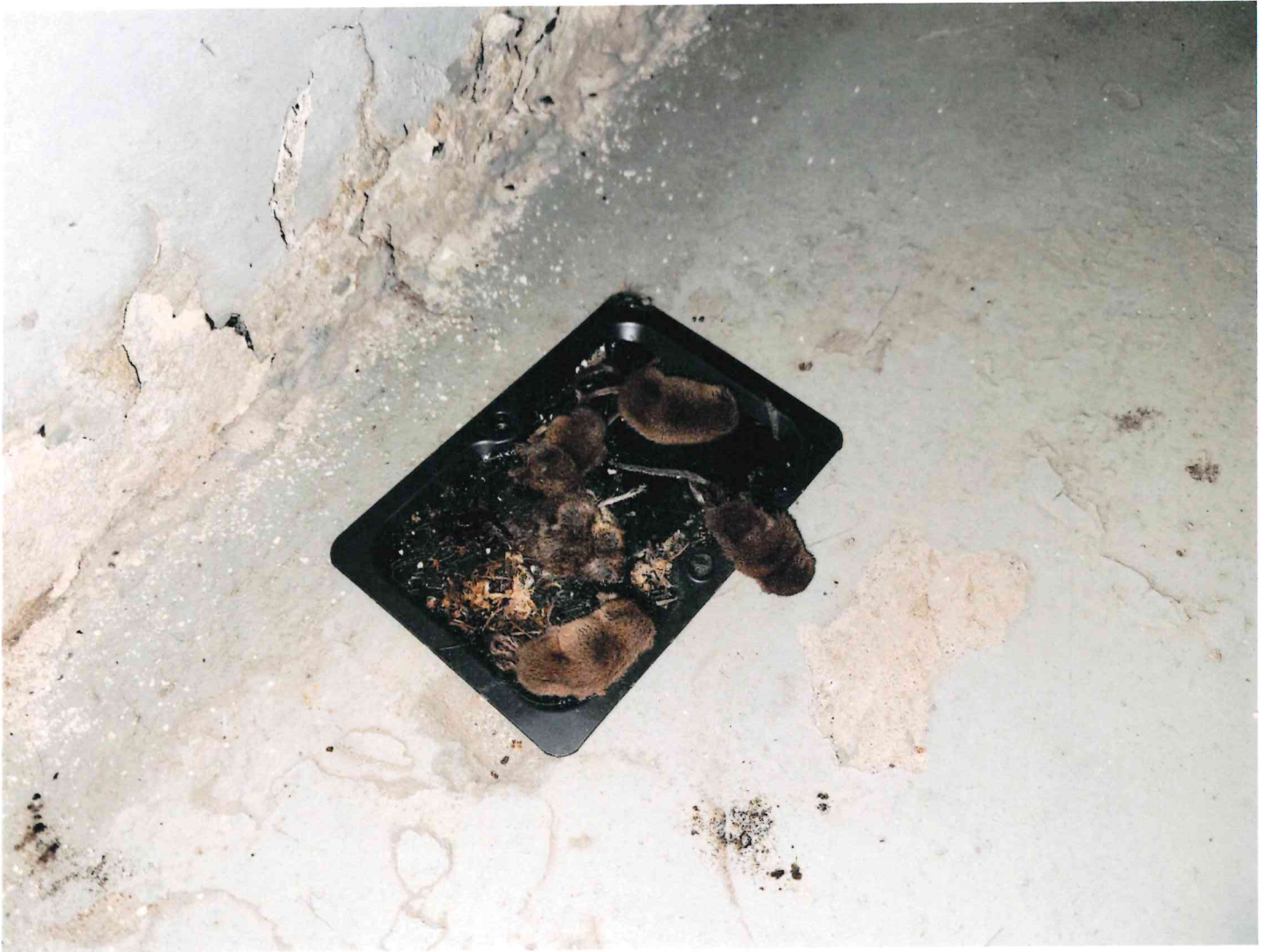
Photo 7: Dead mice and mouse droppings throughout the building.
