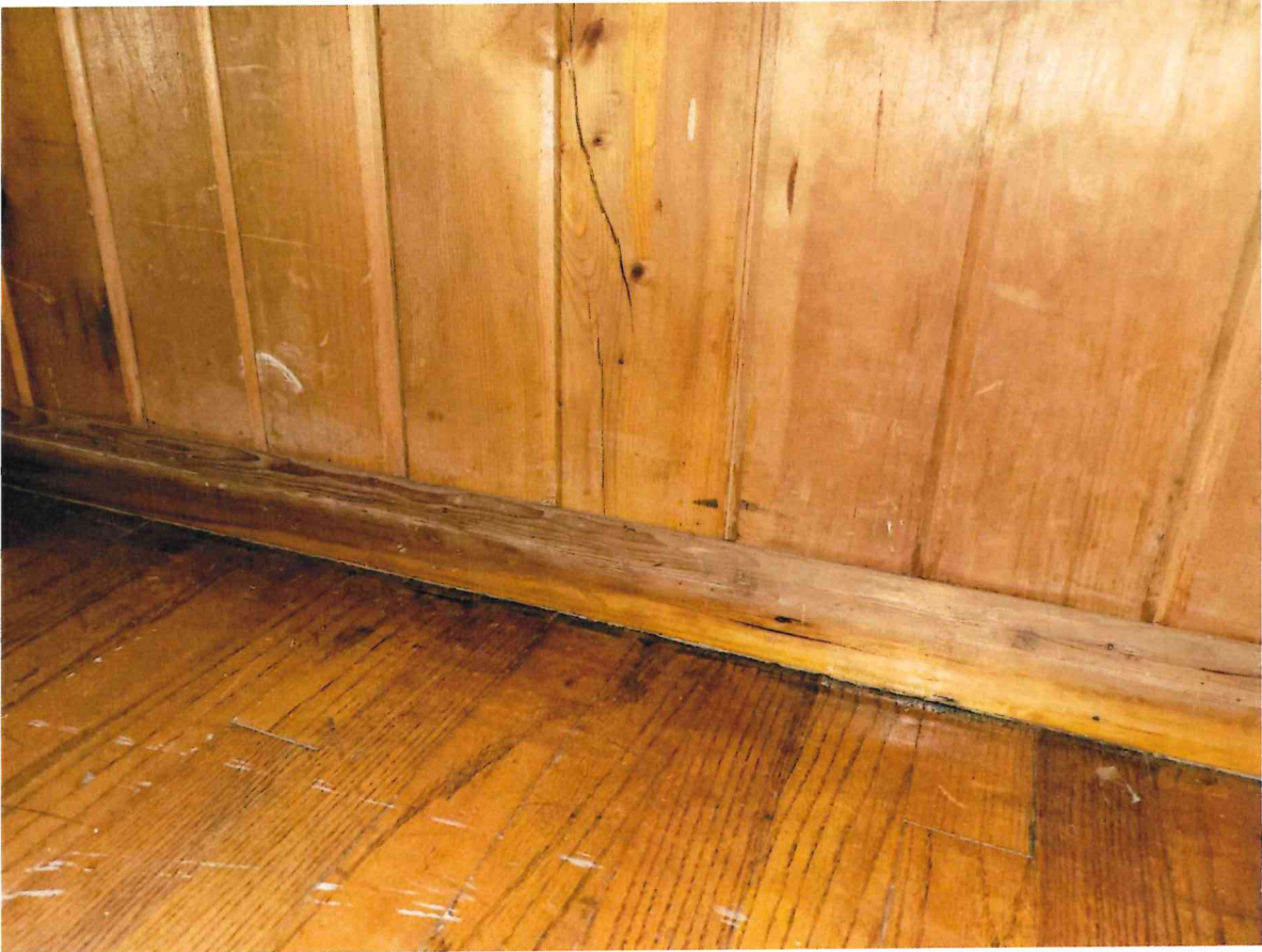
Photo 6: Visible water damage and spotting on wood walls and baseboards on the stage.
