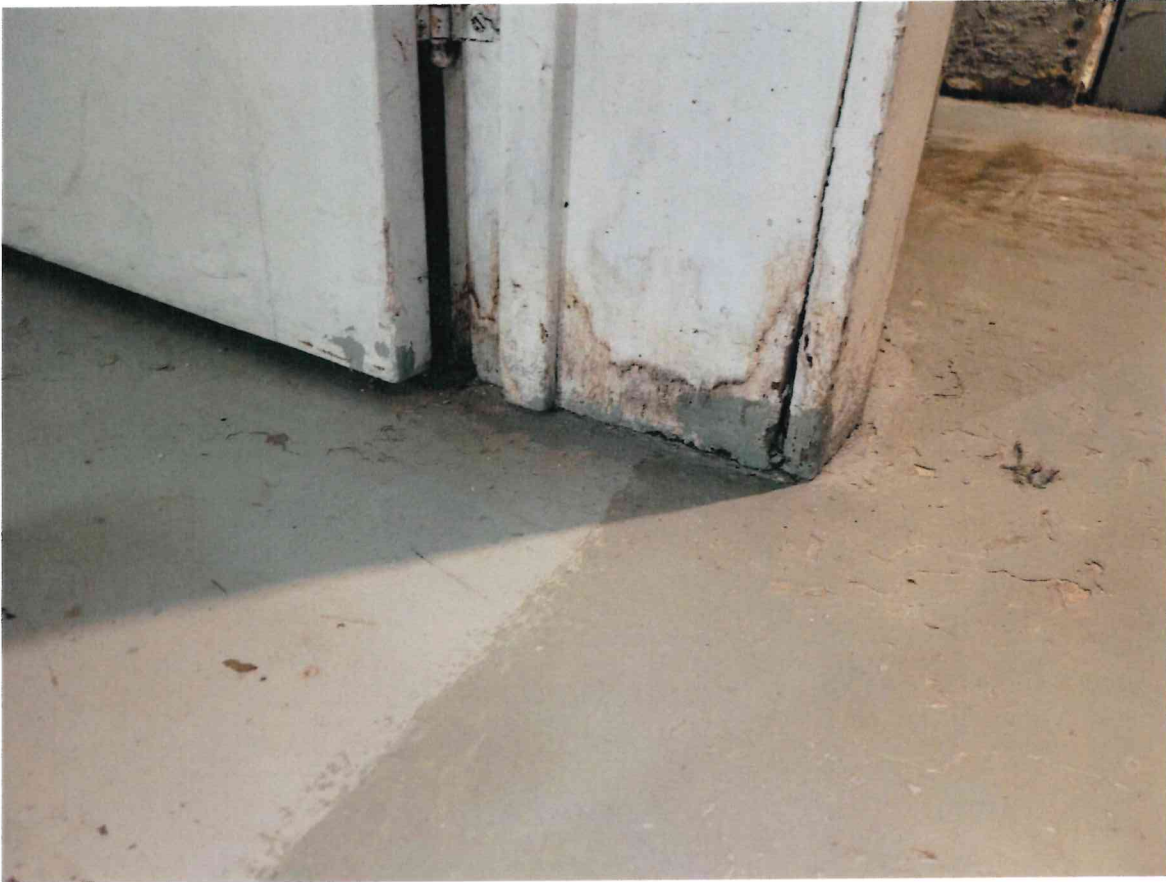
Photo 5: Visible water damage and spotting on wood door frames throughout the basement.
