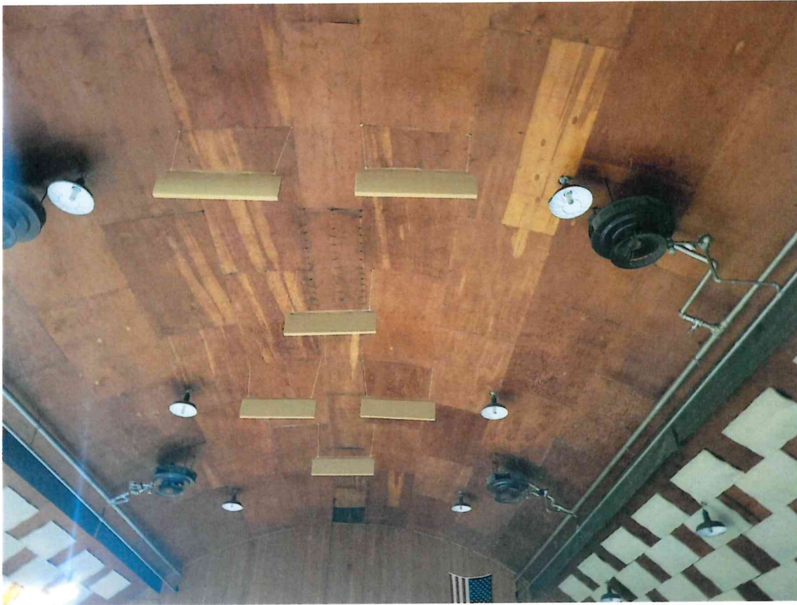
Photo 1: Visible water damage and spotting on the wood ceiling in the gym.
